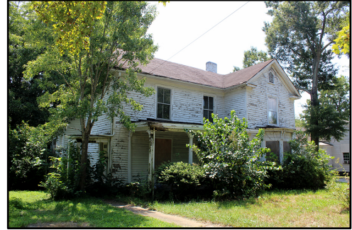
Figure 30: Bradsher House (VN0303) Abandoned and overgrown, the house suffers from deferred maintenance.
