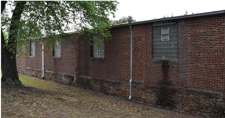
The oldest section of the Pineburr Mill (BK0652, SL 2023) sits on a stone foundation. Photo by author.
