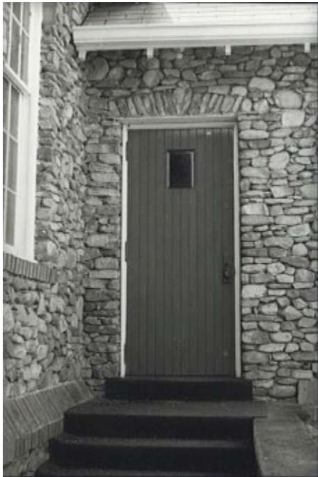
Stonework at the Nebo United Methodist Church (MC0157). Photo by Ted Alexander, 1985. MC0157 Nebo United Methodist Church Survey File, Western Regional Office File Room, North Carolina State Historic Preservation Office, Asheville, NC.
