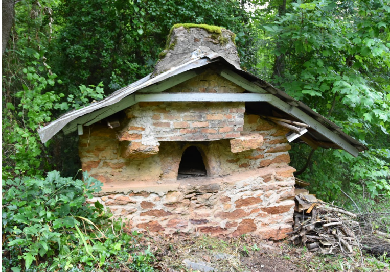
The Albert Pons Bake Oven (BK0482, SL 2022) has a stone base, arched oven opening, and gable roof. Photo by author.
