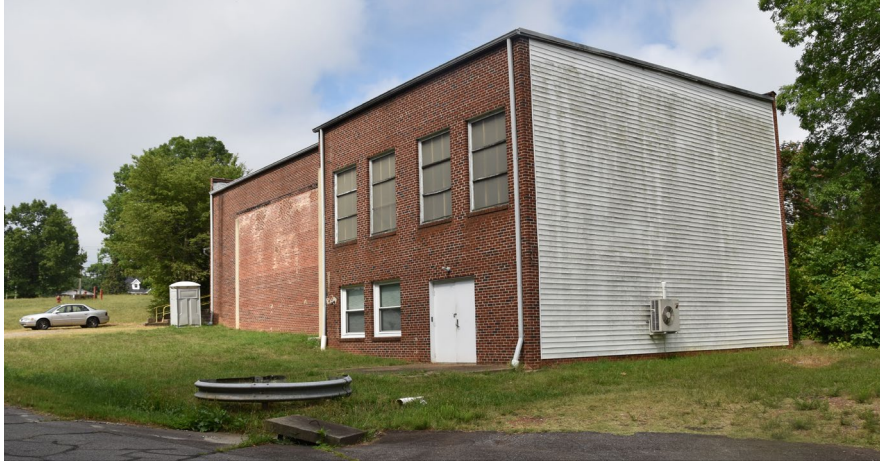
Vinyl cladding can be seen on the rear of the Francis-Louise Full Fashion Mill (BK0453). The building also has replacement windows and some sort of fenestration changes indicated by the change in brick. Photo by author.
