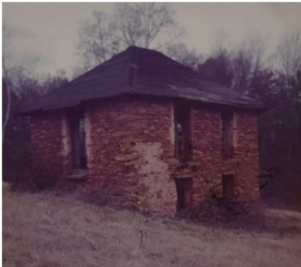
A banked stone outbuilding at the Jean-Pierre Ribet House. Land now owned by Alba-Waldensian. Photo courtesy of the Waldensian Heritage Museum Archives, Valdese, NC.
