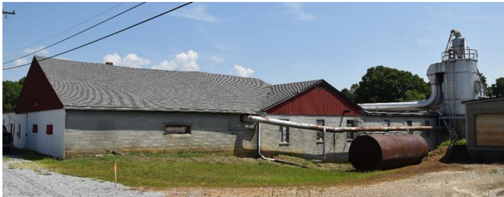
Figure 48. The original section of the Ideal Frame Company (AX0164). Photo by author.
