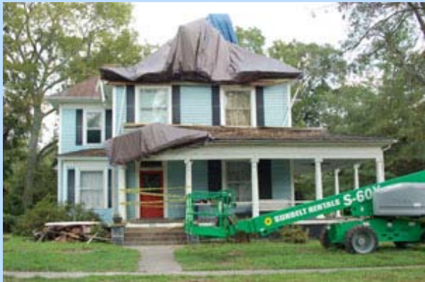
Hurricane Irene damage to the former Presbyterian Manse, Tarboro
