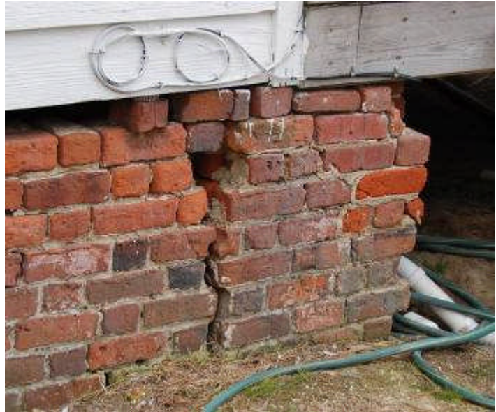
Structural Crack in Foundation Pier
