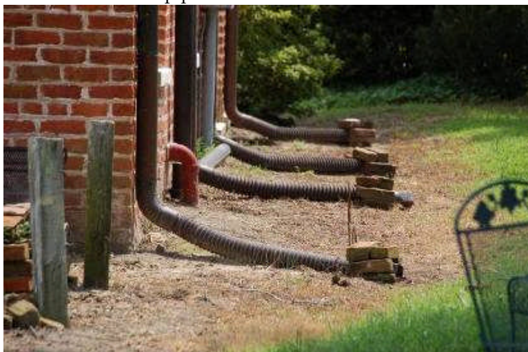
Temporary corrugated extensions added to downspouts and held in place with bricks to carry water away from a building.
