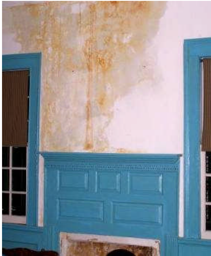
Water Seepage/Damage through Chimney (Hurricane Irene)
